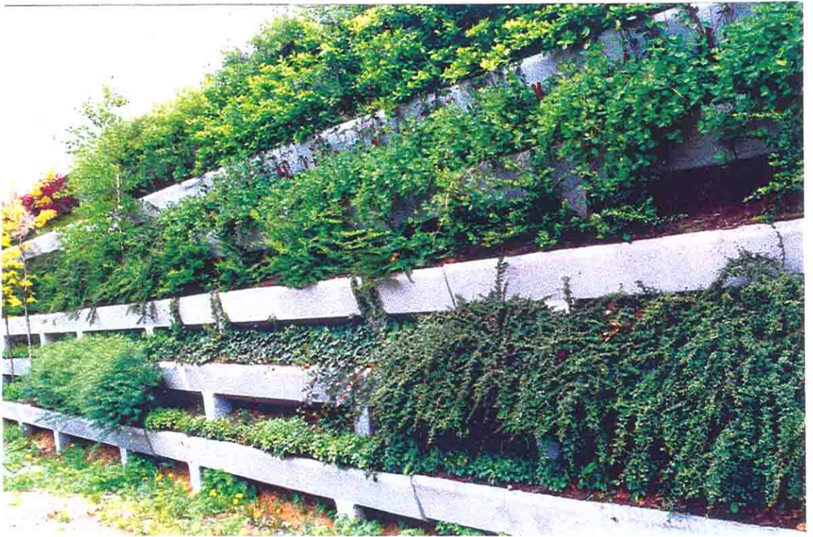
Above-- NYSDOT EVERGREEN NOISE WALL Route 495, Melville, New York
