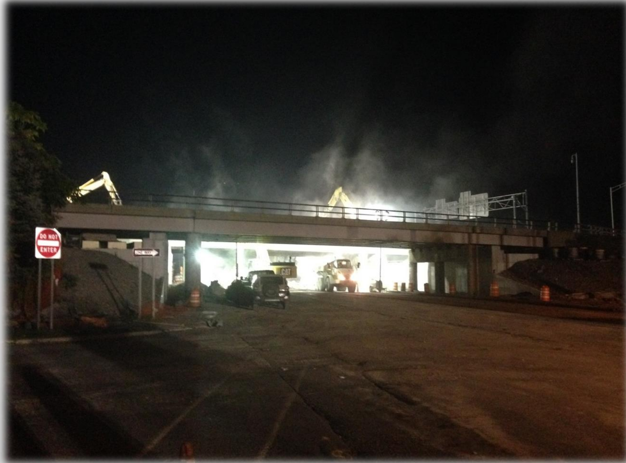
D262260 - I 190 Over Buffalo Ave. Niagara Falls, NY - 72 hr. Bridge Demo & Install
