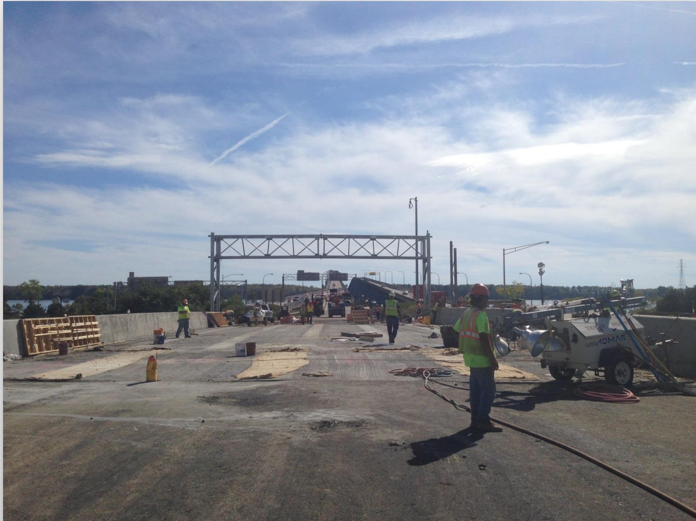
D262260 - I 190 Over Buffalo Ave. Niagara Falls, NY - 72 hr. Bridge Demo & Install
