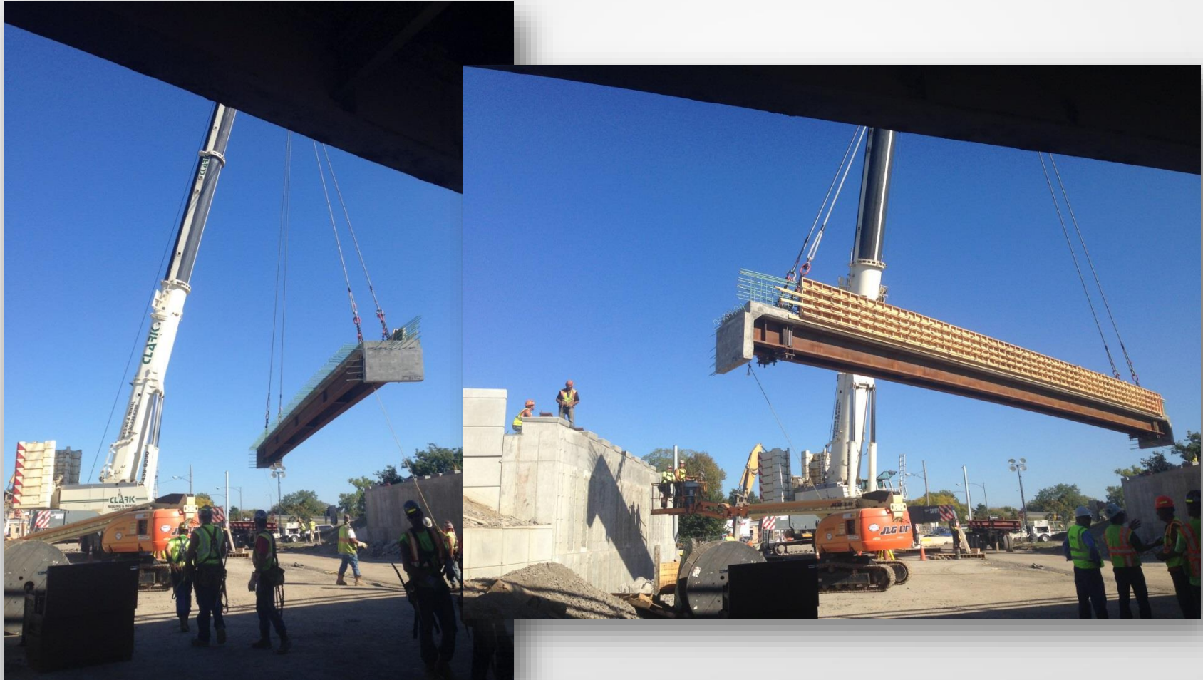
D262260 - I 190 Over Buffalo Ave. Niagara Falls, NY - 72 hr. Bridge Demo & Install
