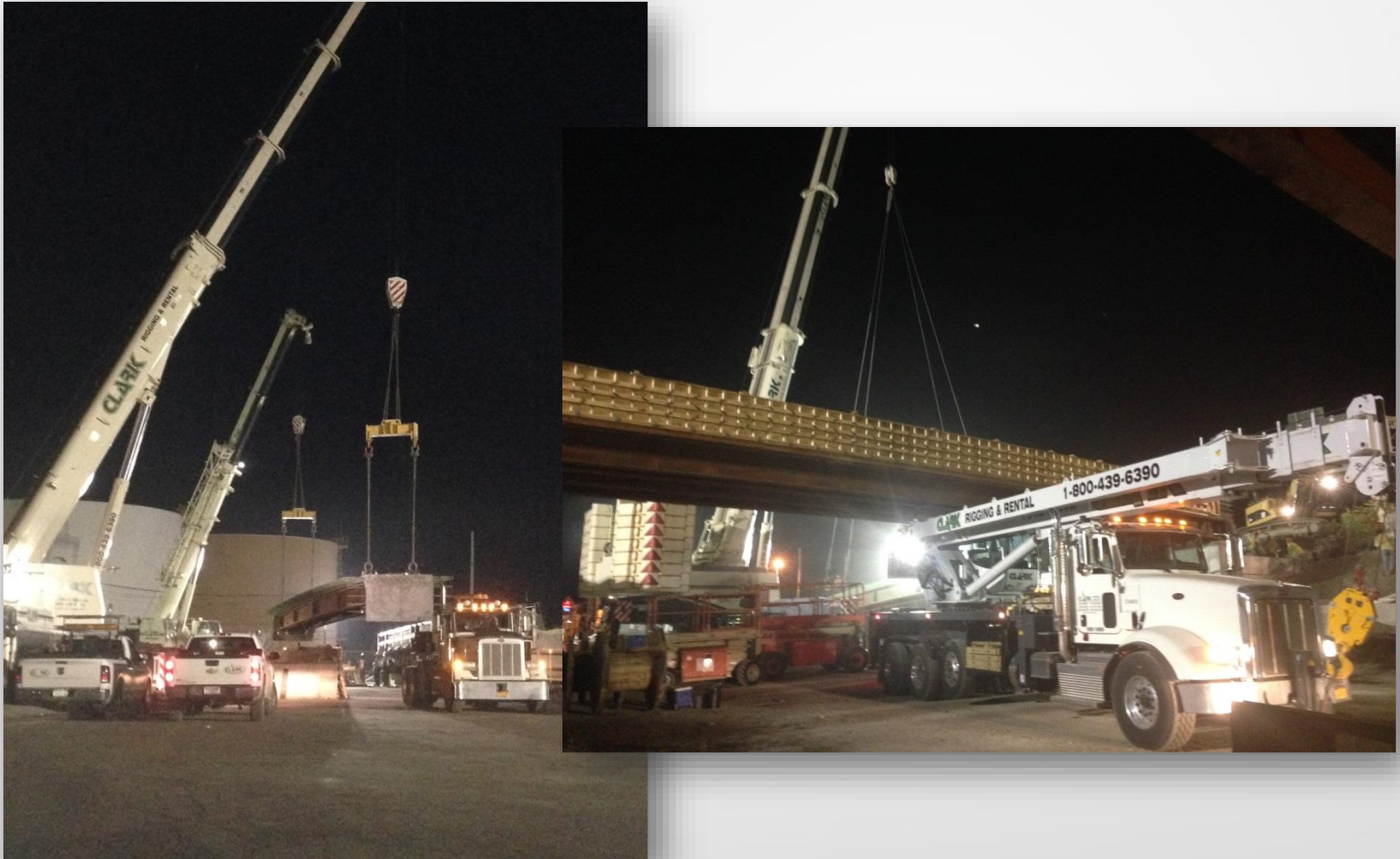
D262260 - I 190 Over Buffalo Ave. Niagara Falls, NY - 72 hr. Bridge Demo & Install
