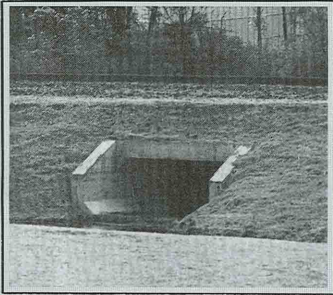
Precast Concrete carries Conrail track in Erie County. Photo by Kistner Concrete
